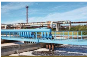
Factory drainage For monitoring final discharge water
