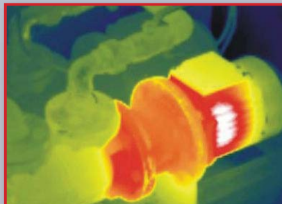
An IR image of a water pump's motor
