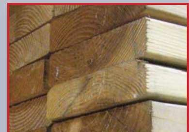
Check wood for dampness or rot
