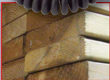
Check wood for dampness or rot
