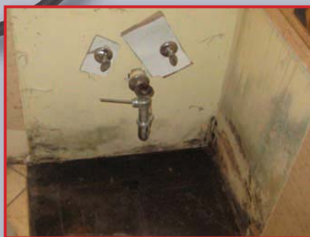
Locate moisture/water damage
