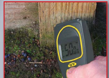
Check wood for dampness or rot
