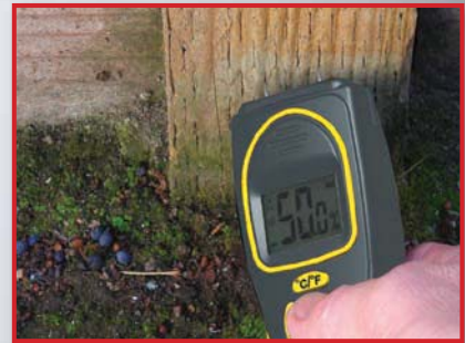
Check wood for dampness or rot
