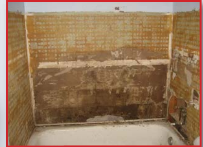
Wet drywall behind removed bathtub tiles
