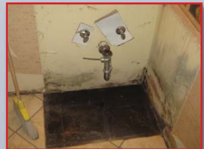
Locate moisture or water damage
