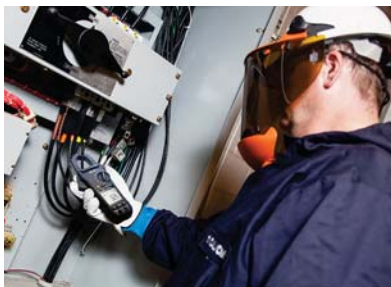
Analyze Power-related Issues
