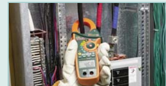
Collecting current measurements and associating them with the right component identified on an infrared image, can be a complicated and cumbersome process
