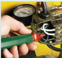
Control panel troubleshoot
