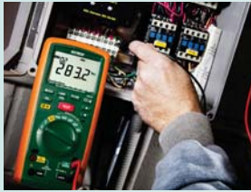
Voltage check on motor starter
