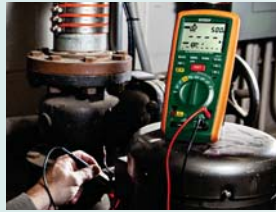
Insulation test on pump motor
