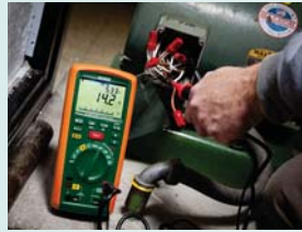
Insulation test on pump motor
